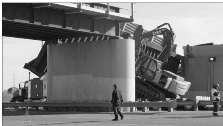
October 11, railway overpass collapses in Lloydminster.
